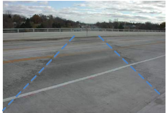
Figure 15 Bridge deck showing ECC link-slab (between dashed lines) after bridge re-opened to traffic
