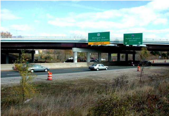
Figure 14 Application of ECC on deck retrofit of a highway bridge in Southeast Michigan
