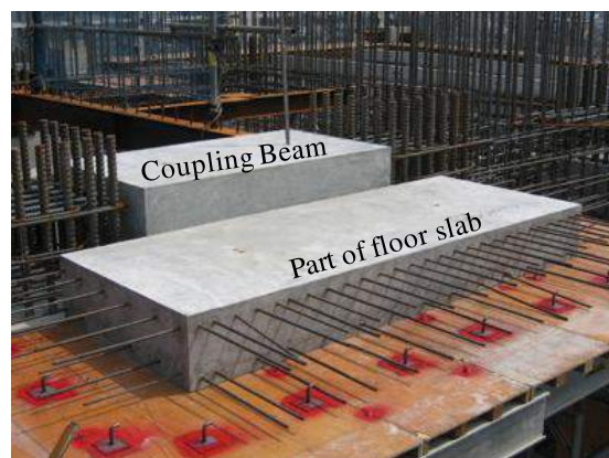
Figure 19 Precast ECC coupling beam dropped into location during building construction (Kanda et al., 2011)
