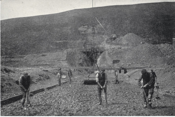
Image 3. Construction at the Talla Dam site, circa 1900. The photo shows the method for cutting the layers of clay in the puddle trench. A skip lowered from "The Blondin" (a cableway) can be seen in the background. The Clay was placed in layers; the compaction of the clay (known as puddling) was completed by hand.
