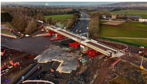
Aerial of the new bridge in final position with four SPMTs underneath. Credit: Skanska
