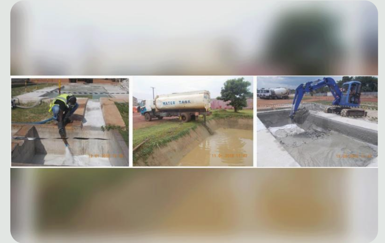
Sedimentation & lime-neutralisation pond for concrete waste.
